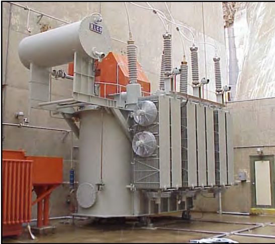
Figure 1 – Typical GSU Three-Phase Transformer.
