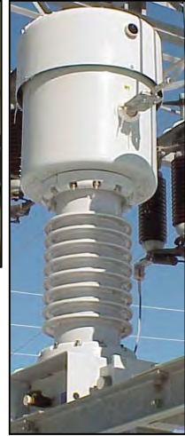
Current Transformer in Switchyard.
